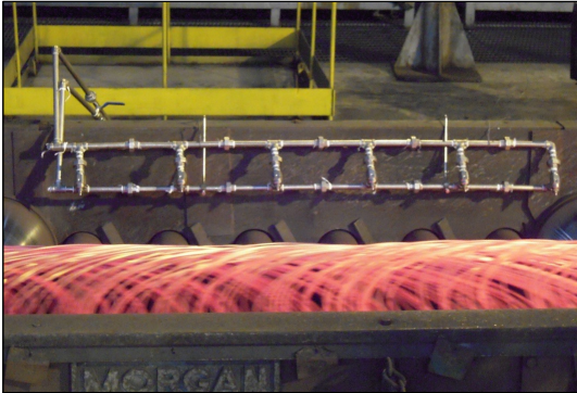
Fig.8. The developed mist cooling system was installed on the Stelmor cooling bed.
